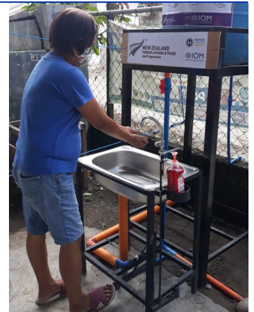
An IOM-installed handwashing station in Magsaysay, Davao del Sur, Philippines, helps IDPs practice proper hand washing. ©IOM, 2020
